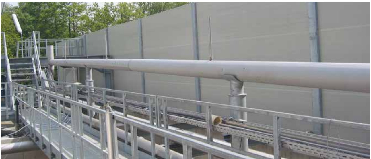
Noise panels at chemical plant, Luneville, France.
