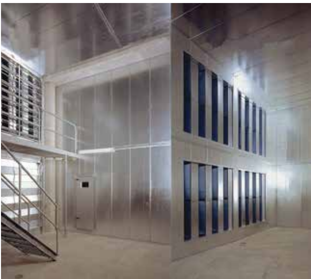
Noise attenuator, fan room, Kista Entre, Stockholm, Sweden.
