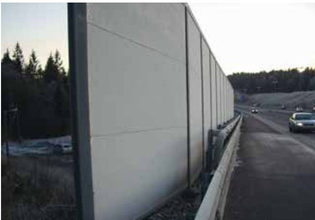
Aluminium noise panels, resistant to salt, along highway E6, Mossporten, Norway
