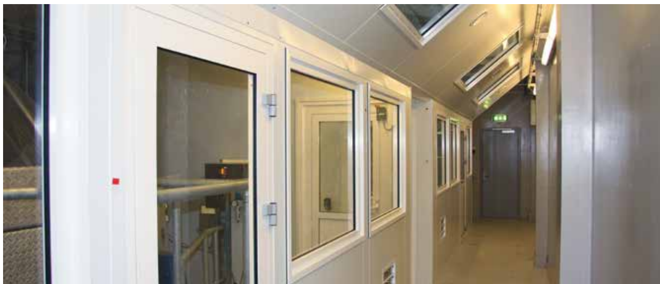
Enclosures/partitions at production facility, Novozymes A/S, Bagsvaerd, Denmark.
